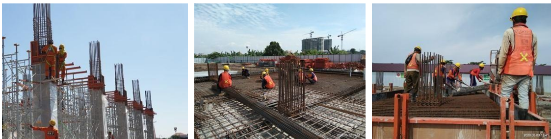
Fig. 2. The molding process, steel reinforcement, and casting process in the construction site (UINSA Surabaya)
