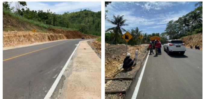
Fig. 1. The recent road development in the south coast of the East Java region
